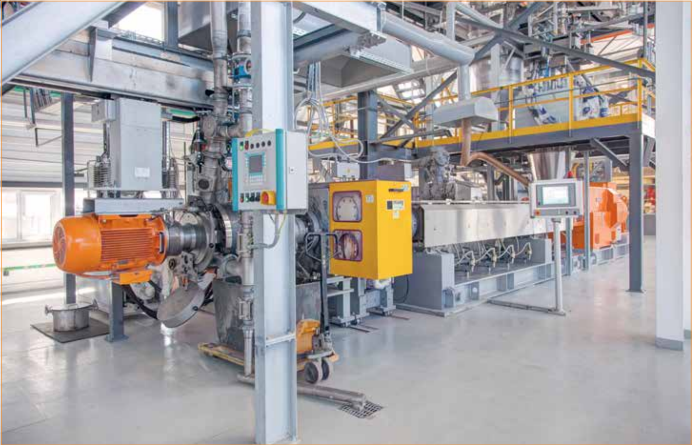
Compounding line with a ZSE 180 MAXX and underwater pelletizing system
